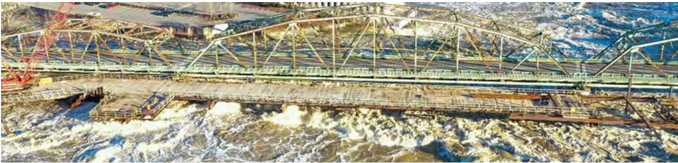
Frank J. Wood Bridge in Topsham during the December 2023 storm. The bridge was closed during the storm due to safety concerns. Photo: D. Scrapchansky, courtesy of the Town of Topsham
