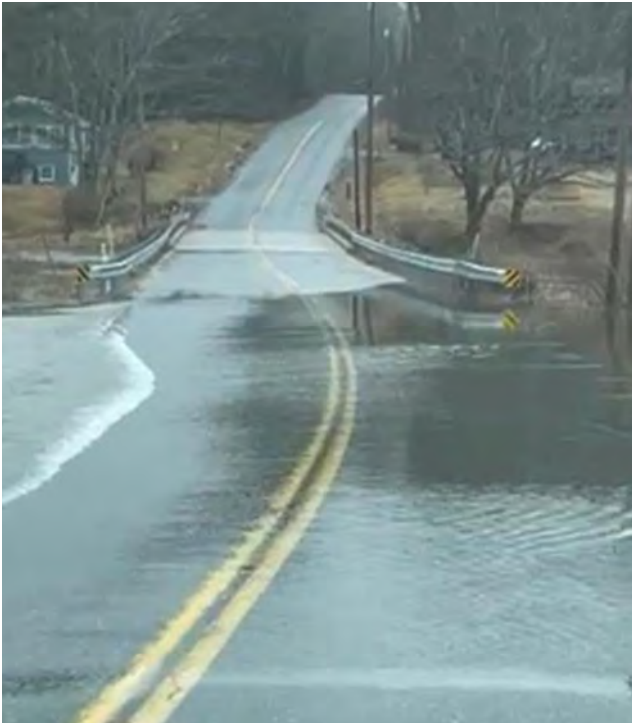
Flooding on the Foreside Road Bridge during a recent storm. Photo courtesy of the Topsham Public Works Department.
